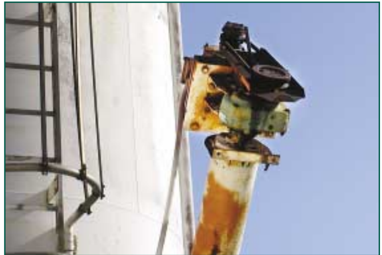
Conveyor motor and belt need cover
