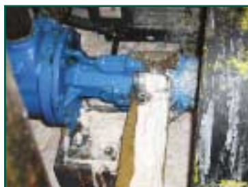
Leaky gear packing
