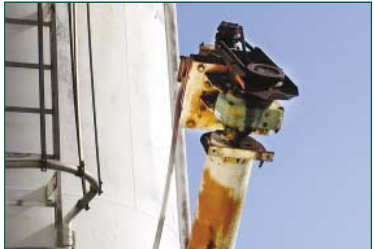
Conveyor motor and belt need cover
