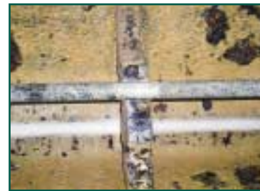
Center bearing missing
