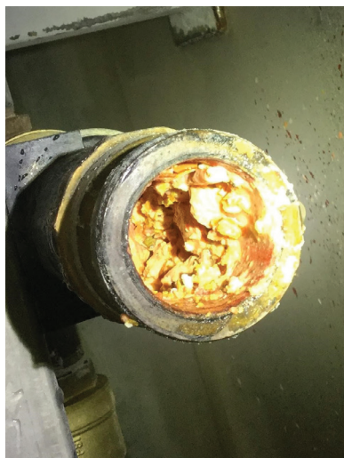
PLUGGED STARCH LINE
