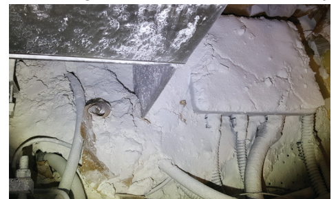
Accumulation of borax dust in hopper area
