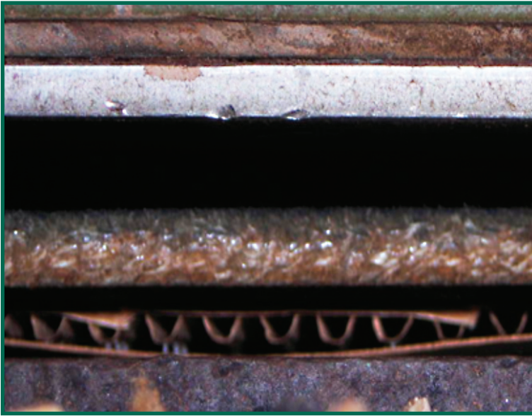
Here the board is pulling apart at the double backer; the bond is irretrievably lost.
